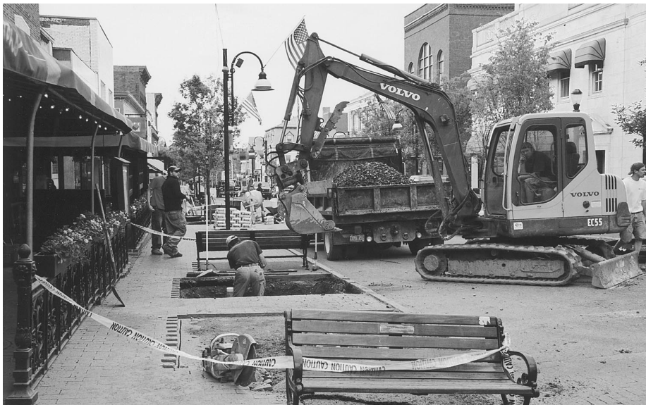
Keeping downtowns strong means keeping them attractive. Here, new trees and paving are being installed along Burlington, Vermont's main downtown street.
